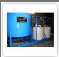
Auto pH Controlling (Neutralisation) System
