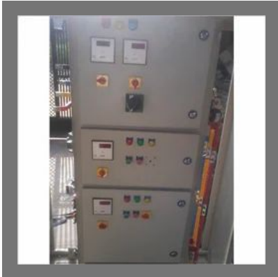
Electrical Fire Fighting Panel
