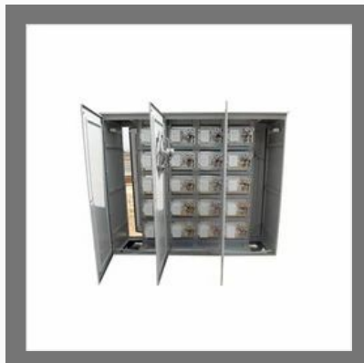
Feeder Pillar Panel
