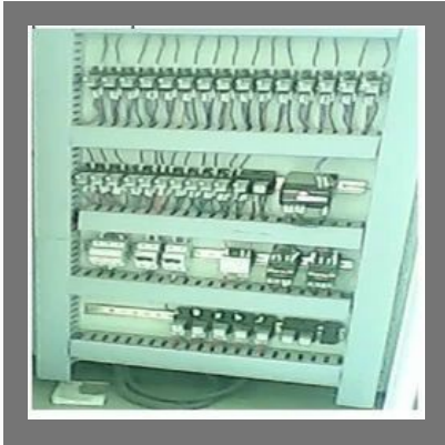
Relay Control Panel
