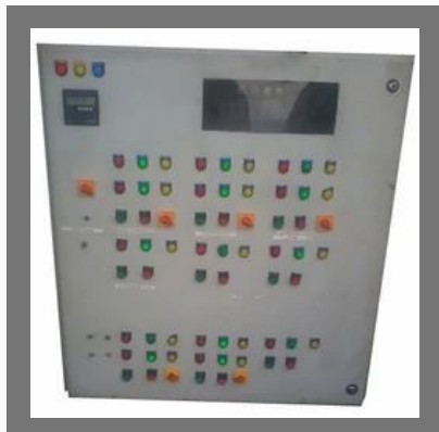
STP Control Panel
