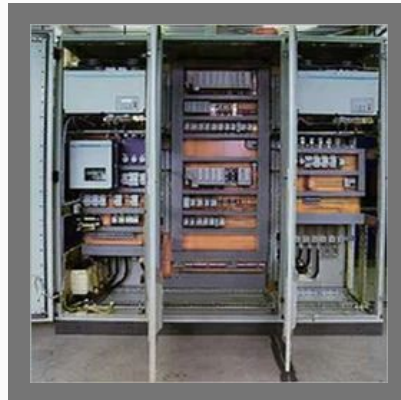
VFD Control Panel
