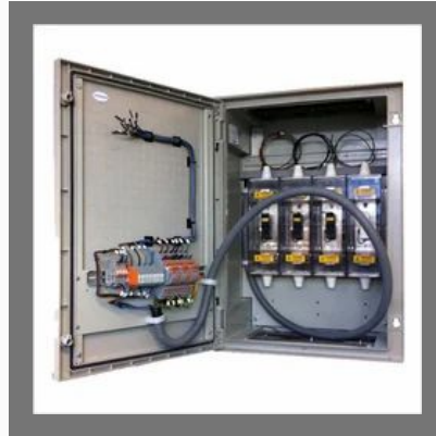
Electric Meter Panel
