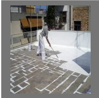
General Waterproofing Services
