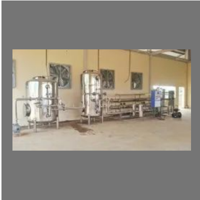
Industrial RO plant
