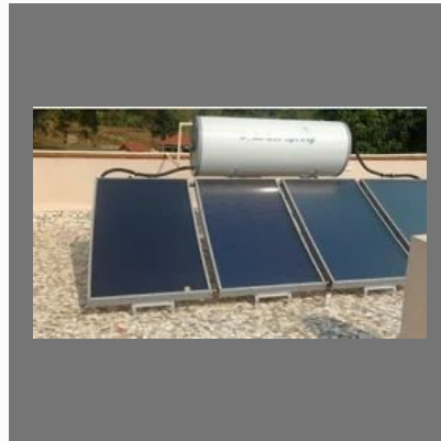
Solar Water Heating System
