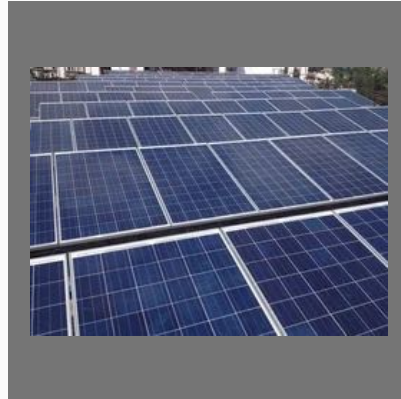
Solar PV Roof Top Solutions
