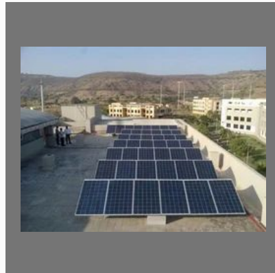
Solar PV Roof Top Solutions
