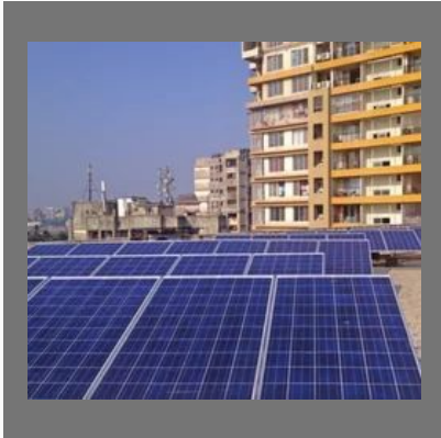
Solar PV Roof Top Solutions
