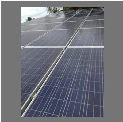
Solar PV Roof Top Solutions
