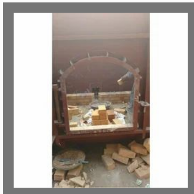
Furnace Refractory Lining
