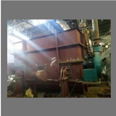
Aluminum Melting Skelner Furnace
