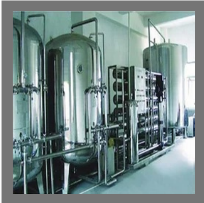
Mineral Water Plant
