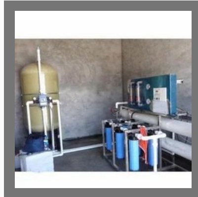
Industrial RO System
