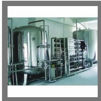
Fully SS RO Plant
