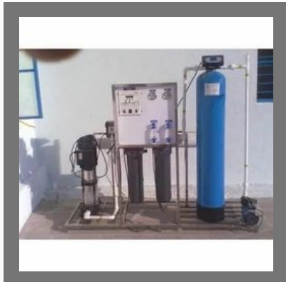
Industrial RO Plant
