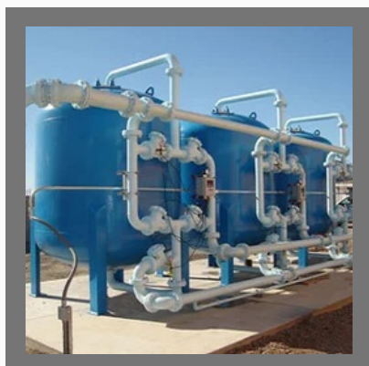
Drinking Water Treatment System
