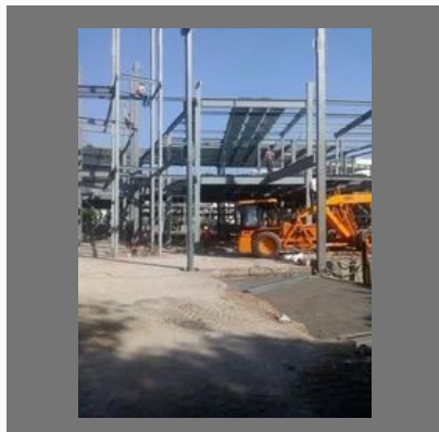
Industrial MS Structure Services
