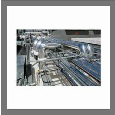
Carrier HVAC System
