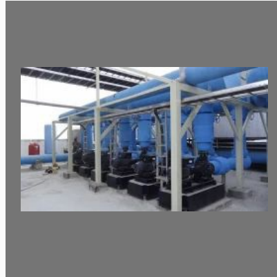
Blue Star HVAC System
