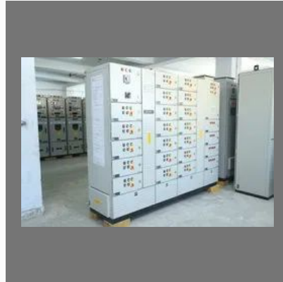
MCC Electrical Control Panel
