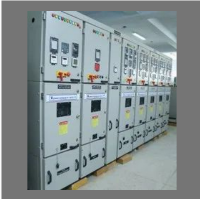
11 KV / 33 KV VCB/HT Panel
