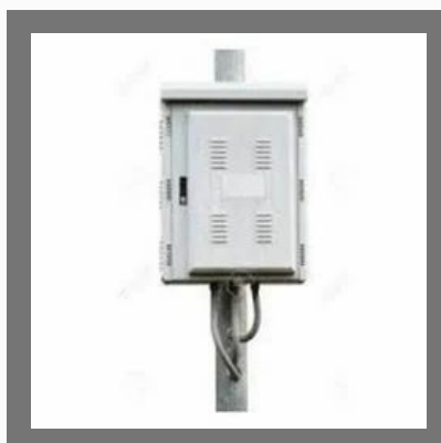
Electrical Pole Box
