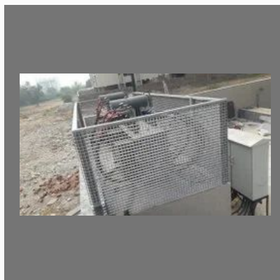
FRP Fencing for Transformers
