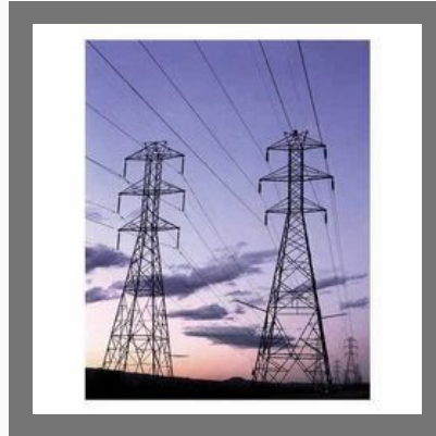
Over Head Transmission Lines
