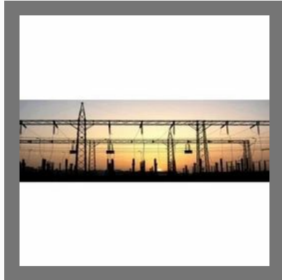
High Voltage Sub-Station
