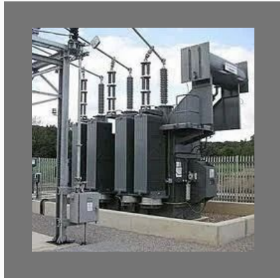
High Voltage Distribution System
