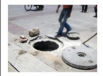
Rainwater Harvesting System
