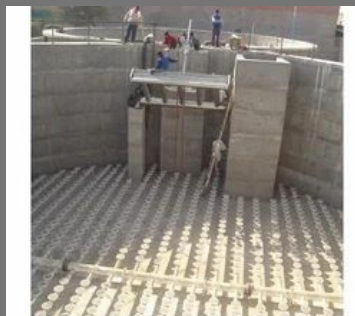
Commercial Sewage Treatment Plant
