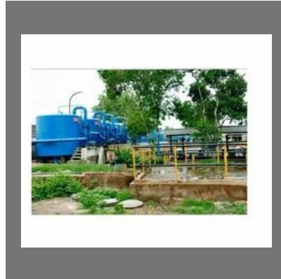
Sewage Water Treatment Plant
