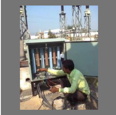
Junction Box & Control Panel Testing
