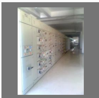
Panel Installation Services
