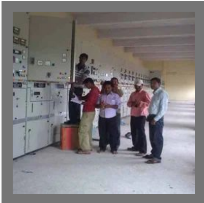
HT Panels And Control Panels Testing
