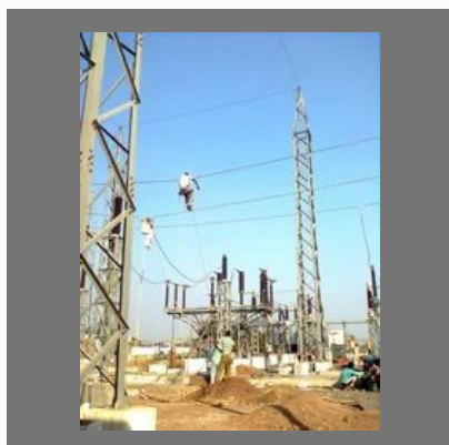
EHV Maintenance Contractors
