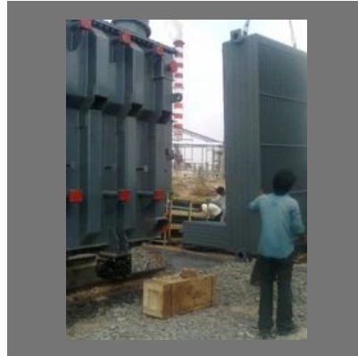
Transformer Oil Filtration & Unloading Services
