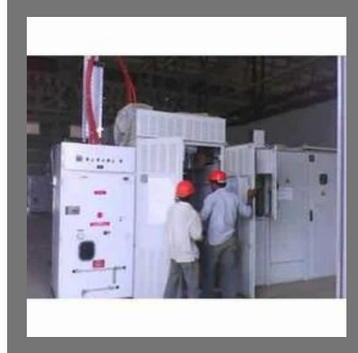
Indoor Type Station Transformer Testing
