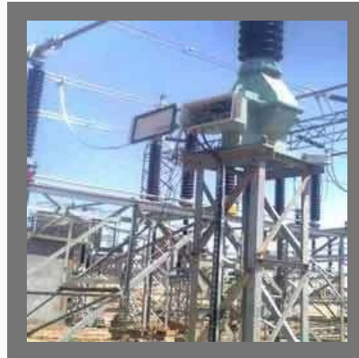
EHV Equipment Testing
