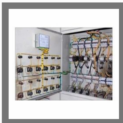
Electrical Control Panel
