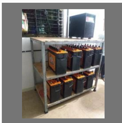
Off Grid Solar System With Battery Back Up System
