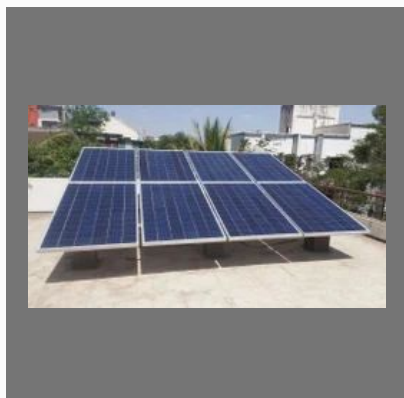
On Grid Solar Power System
