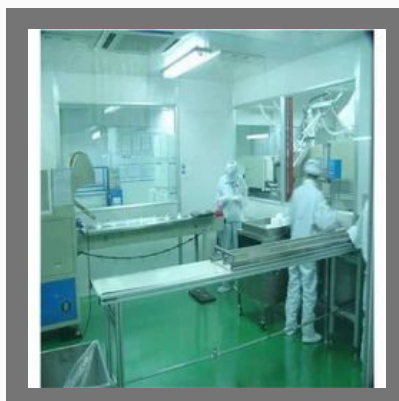
Modular Clean Room
