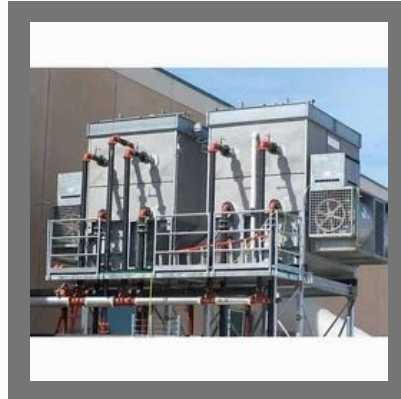
Central Air Conditioning System
