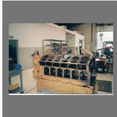
Power Generators Maintenance Service
