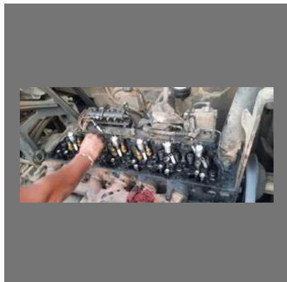
Diesel Generator Maintenance Service
