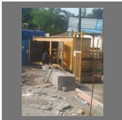
CAT Diesel Generator
