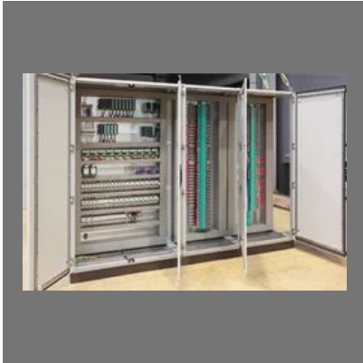
PLC Based Control Panel
