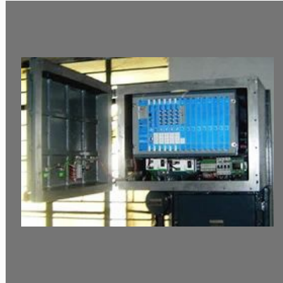
Relay Based Instrumentation Panel
