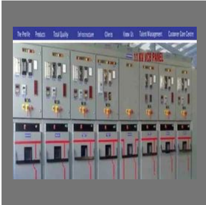
11 KV VCB Panel
