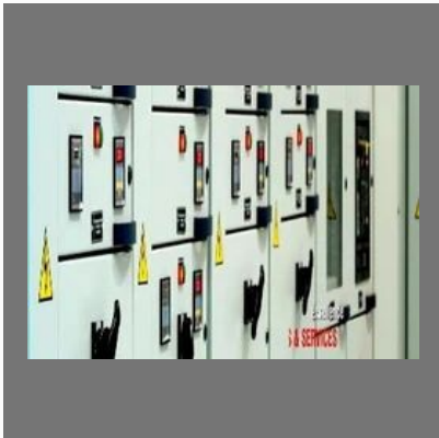
Control & Relay Panel
