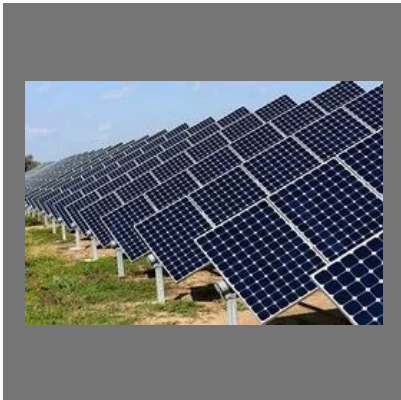
Industrial solar Power Plant
