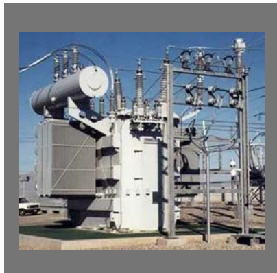
Power and Distribution Transformers
