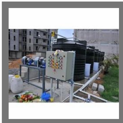
RO Control Panel
