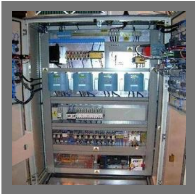
RO Control Panel Maintenance Service
