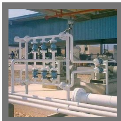
LPG Pipeline Designing Services
