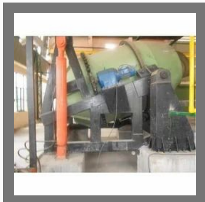
Tilting Rotary Furnace
