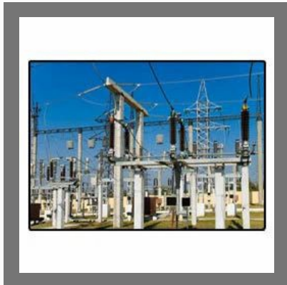
Electrical Equipments Maintenance
