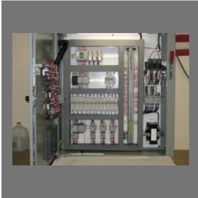
Drives And PLC Panel
