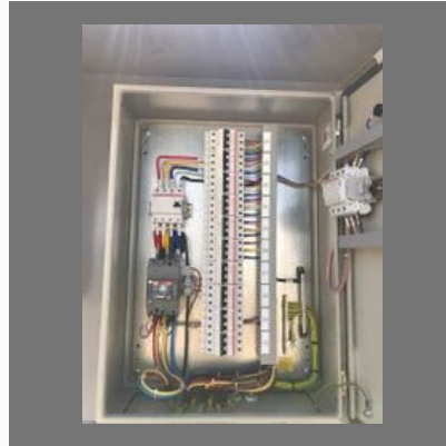
Automation Plc Control Panels
