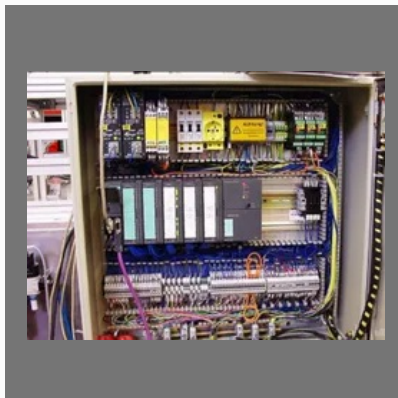
PLC Trouble Shooting Service
