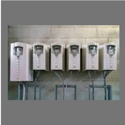
Vfd Installation Service
