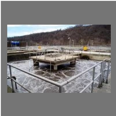
Waste Water Treatment Plant
