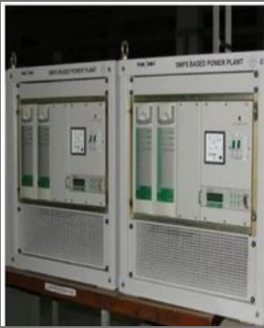
SMPS Power Plant
