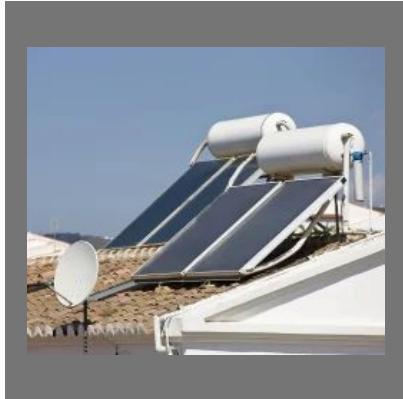
Solar Hot Water Systems
