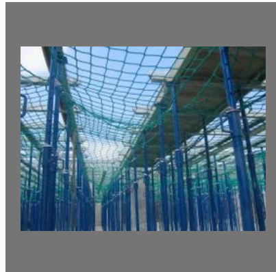
Construction Safety Nets
