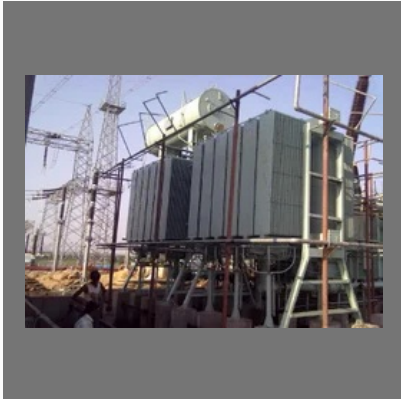
High Velocity & Medium Velocity Water Spray System
