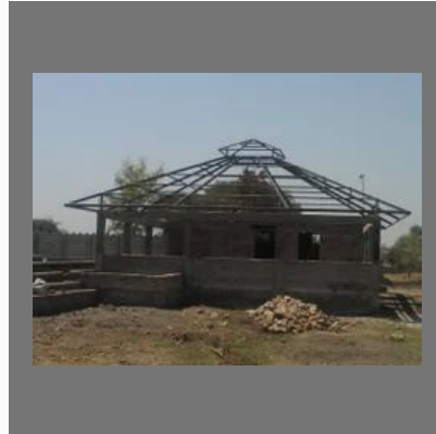
M S Fabricated Structure
