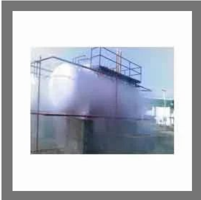
Water Spray System
