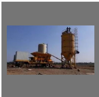
Trailer Mounted Batching Plant
