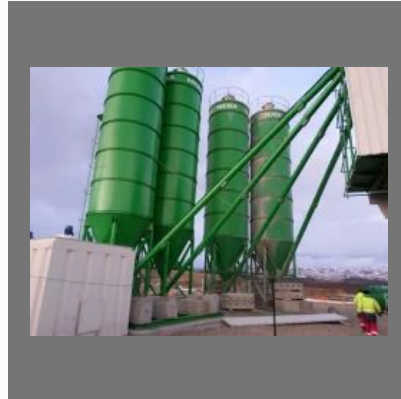
Cement Storage Silo
