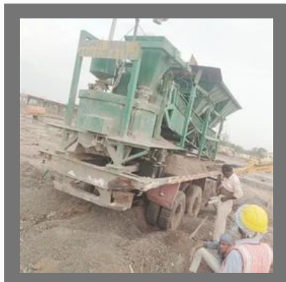
Mobile Concrete Batching Plant
