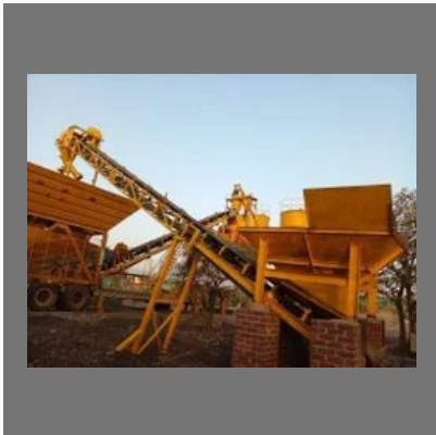
Belt Conveyor System
