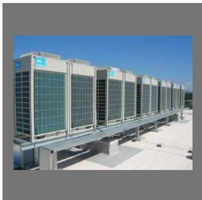
VRF Air Conditioning System
