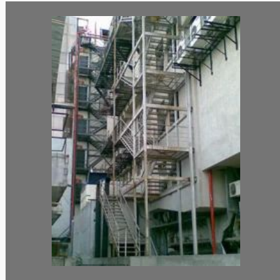
Fire Fighting Staircase
