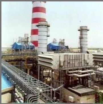
Captive Power Plant
