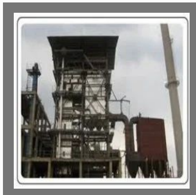
Spent Wash Fired Boilers
