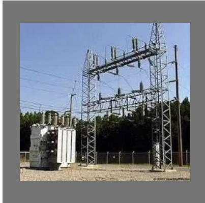
Power And Grid Transformers
