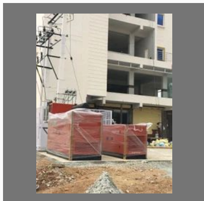
Mahindra Diesel Generator
