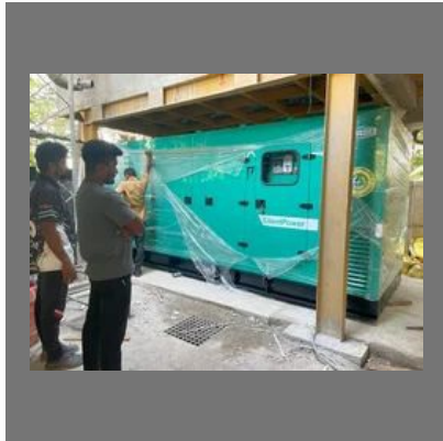
Cummins Diesel Generator
