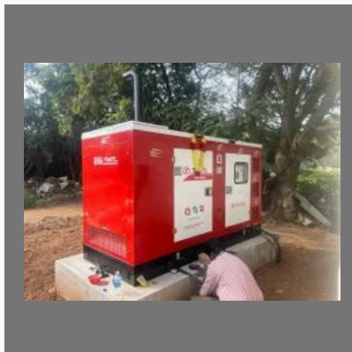
Eicher Diesel Generator
