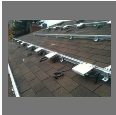
Solar Panel Roof Brackets
