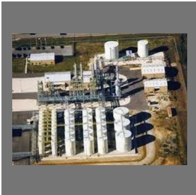
Chemical Storage Tank
