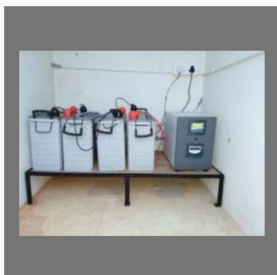
Solar Powered Battery Based System
