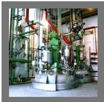
Urea Formaldehyde Resin Plant
