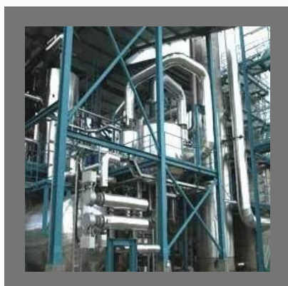
Industrial Formaldehyde Resin Plant
