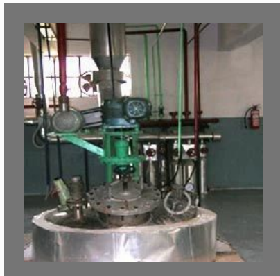
Polyester Resin Plant
