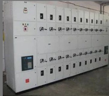
Spinning Mill Change Over Panel
