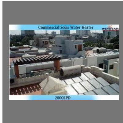
Solar Water Heater
