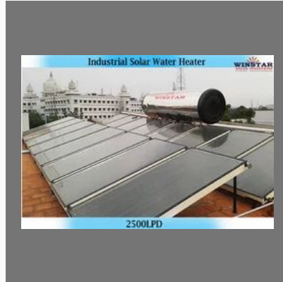
Solar Water Heater
