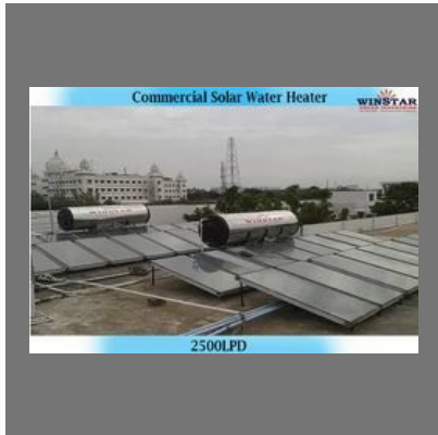
Solar Water Heater
