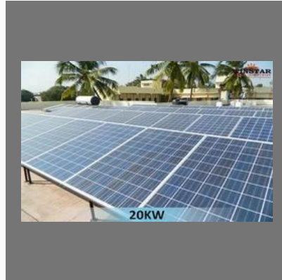
Solar Power System
