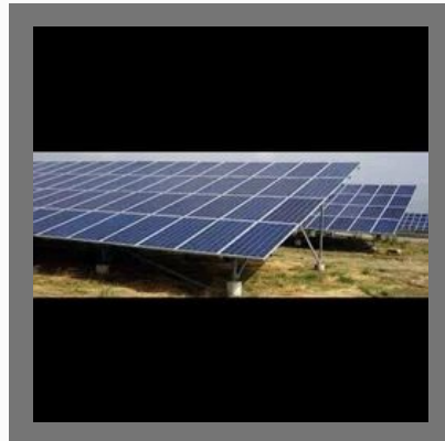
Solar Power Plants
