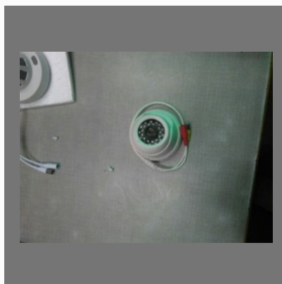
CCTV Dome Camera
