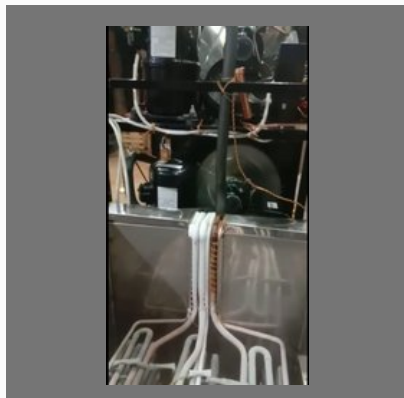
Water Cooling Radiator
