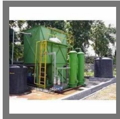
Industrial Sewage Treatment Plant
