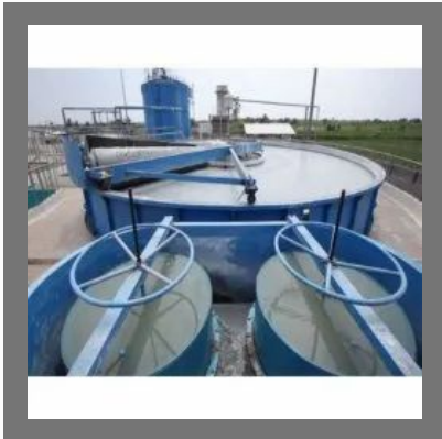
Dairy Effluent Treatment Plant
