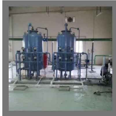
PLC Wastewater Treatment Plant
