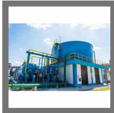
Industrial Waste Water Treatment Plant
