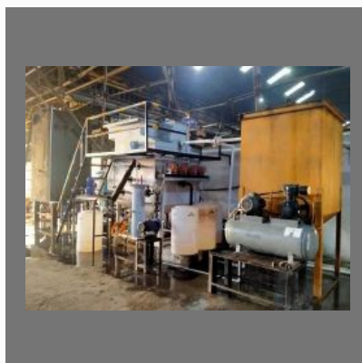
Dissolved Air Floatation Unit
