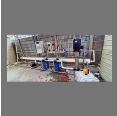
Ultra Filtration and Nano Filtration System
