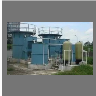
Industrial Effluent Treatment System
