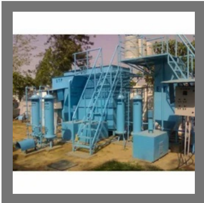
Domestic Sewage Treatment Plant
