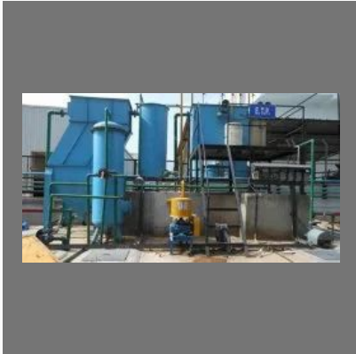
Effluent Treatment Plant
