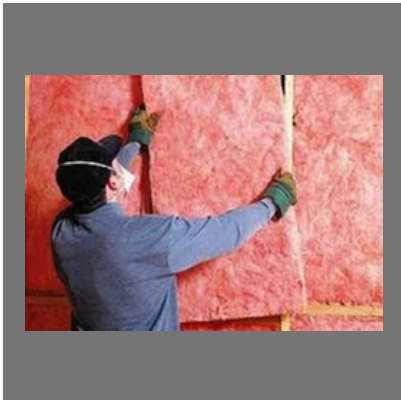
Industrial Maintenance Service
